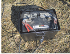
↑ Power cable connected to battery
